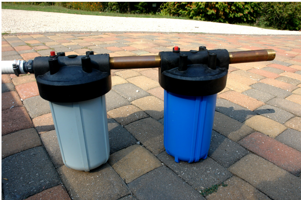
Figure 2. Filter Housing Connections
