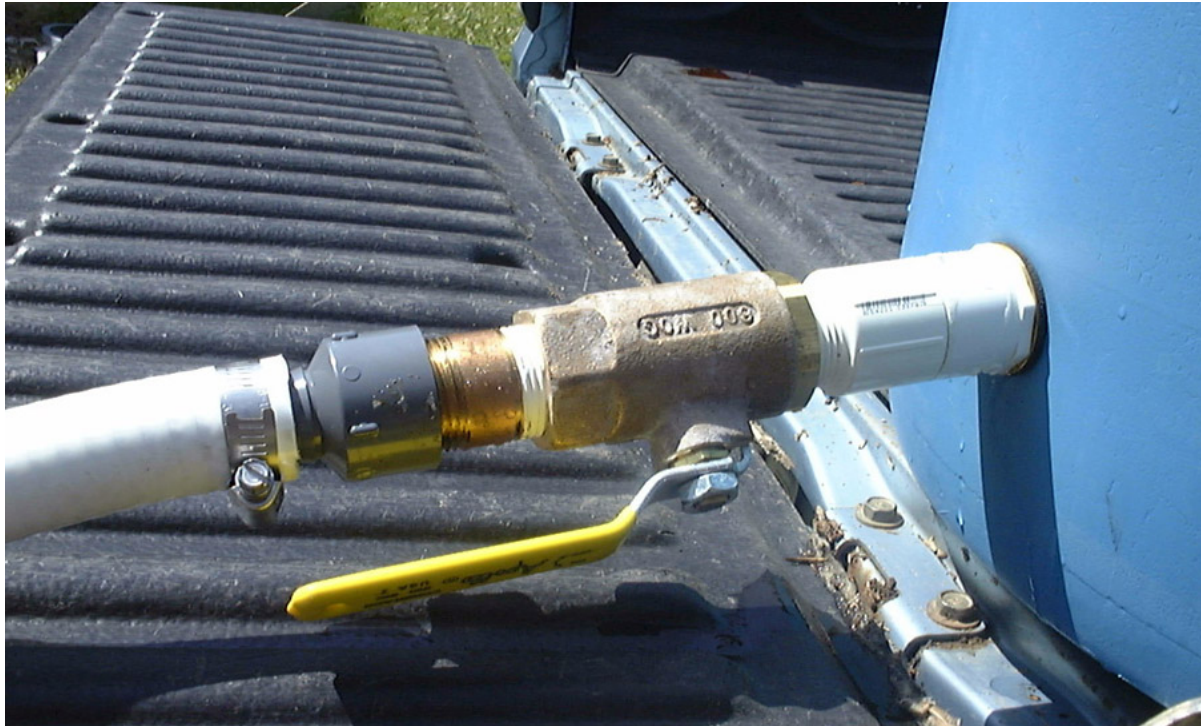
Figure 1. 55-Gallon Drum Connections
