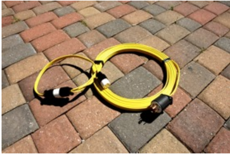
Figure 25. Extension Cord for 220 Volt Water Pump
