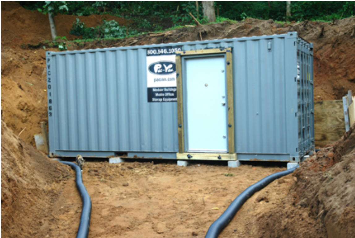
Perforated Drain Tile around Shelter
