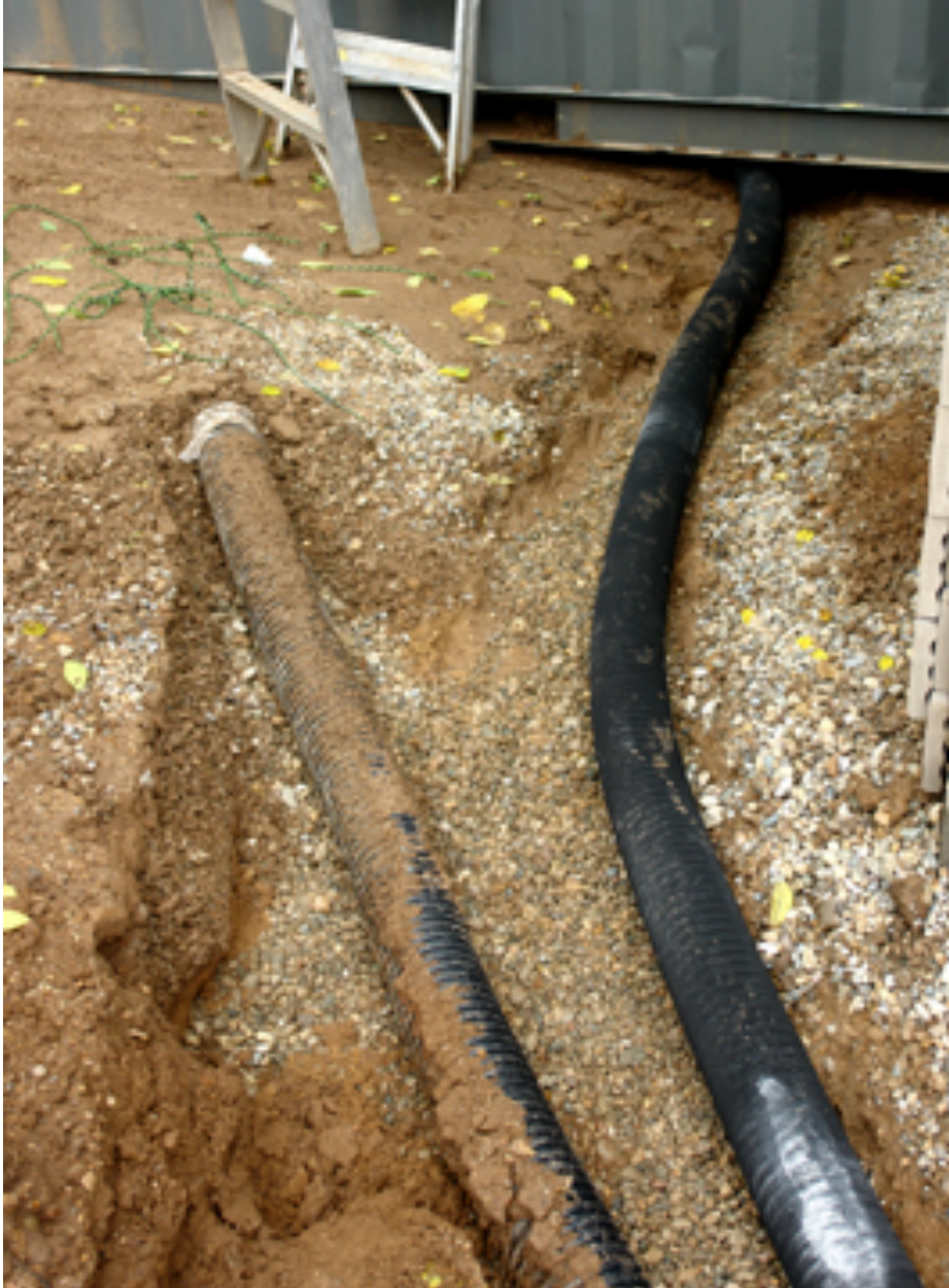
Left - Perforated Drain Tile Covered with Sediment Shield Right - Sock Covered Drain Tile under Shipping Container
