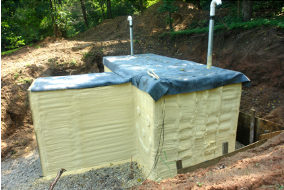
Shelter Covered with Icynene Insulation with Layer of EPDM Rubber Roofing over top
